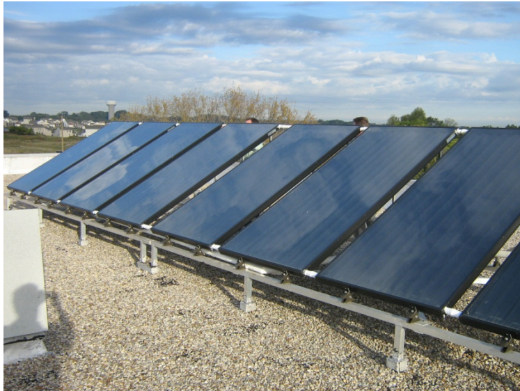
Farmer Elementary Solar Hot Water Panels
