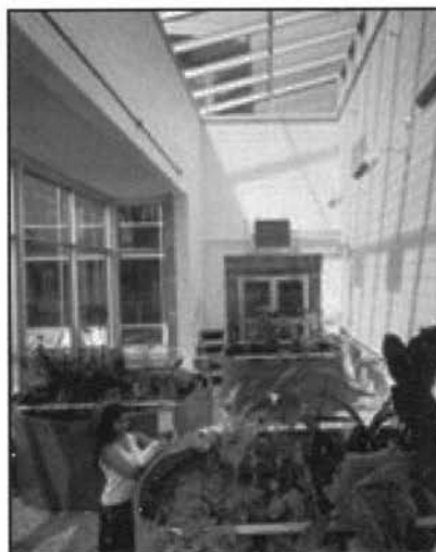
Living Machine used to treat wastewater in the Lewis Center, Oberlin College.
