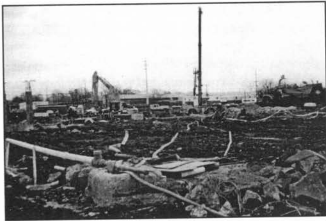
Underground cistern collecting site wastewater
